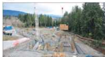
Early stages of the Cascade, a two-building, 153-residence new-home project in Coquitlam.
